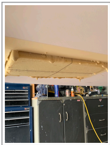
Figure 8 - Protruding High Density Foam on Board Deck
